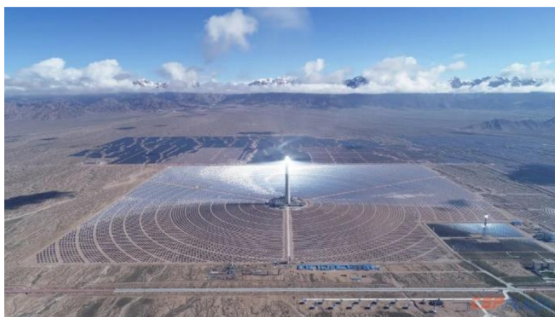
Figure 1 Delingha 10MW Tower Concentrating Solar Power Station
